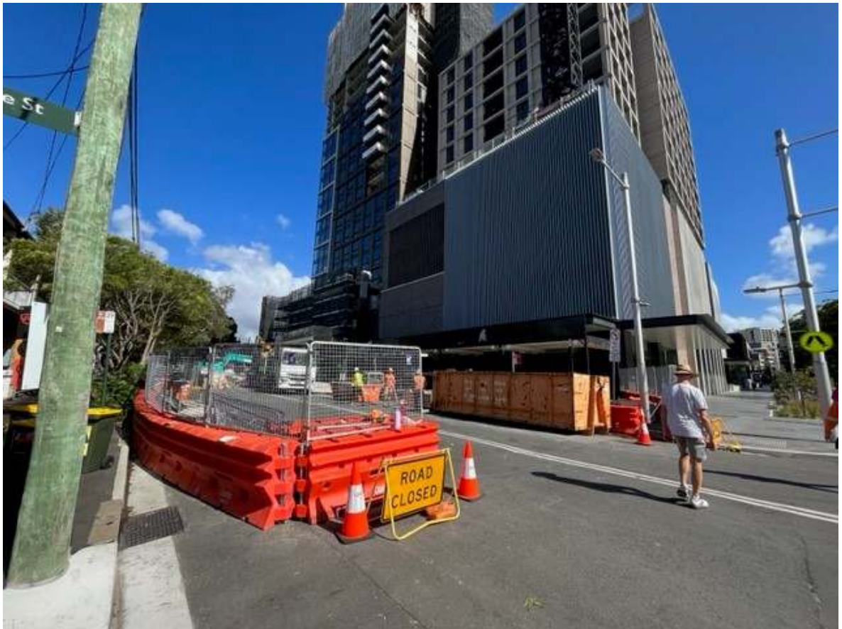
Photo 14: Road closure and work zone on Wellington Street as viewed from the corner of Cope Street.
