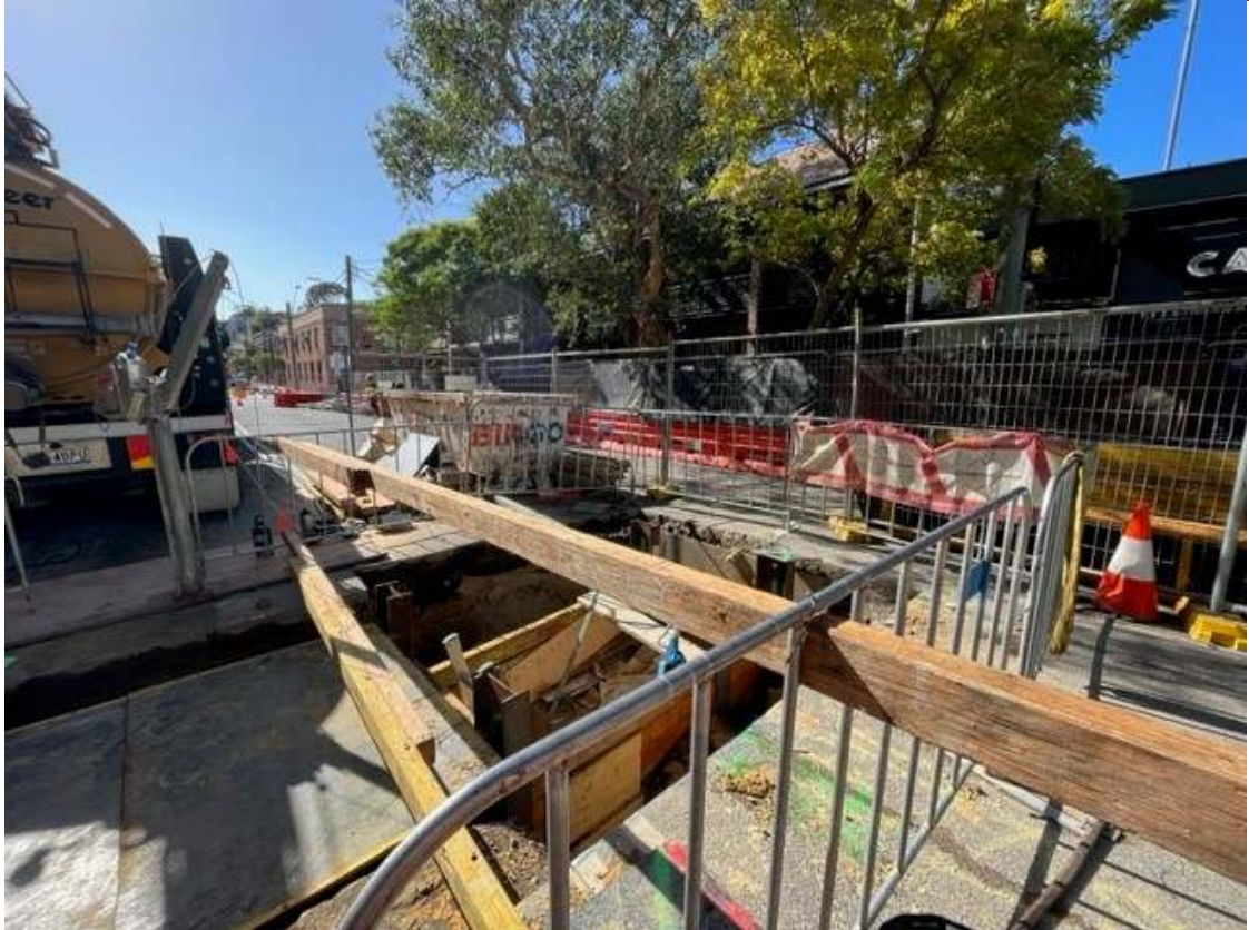
Photos 9-12: A road closure was in place on Wellington Street to facilitate sewer connection works.
