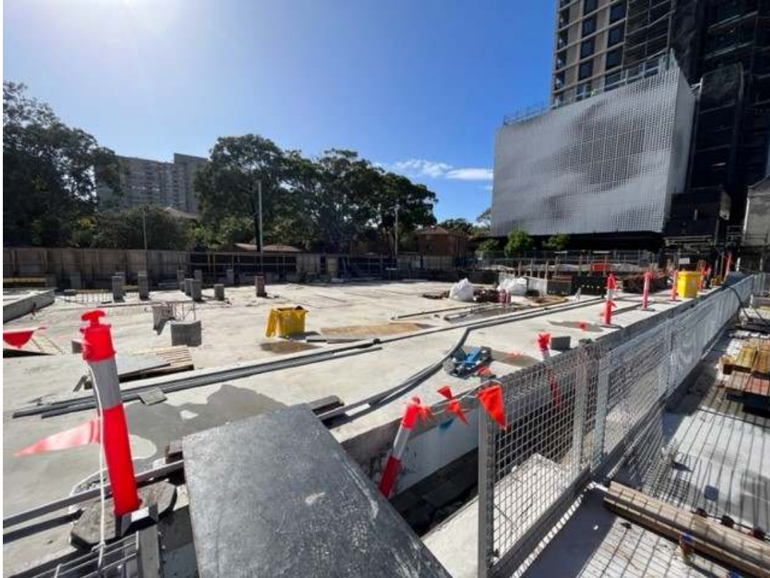
Photos 6 & 7: Site sheds had been removed and works had commenced for Cope Street Plaza.
