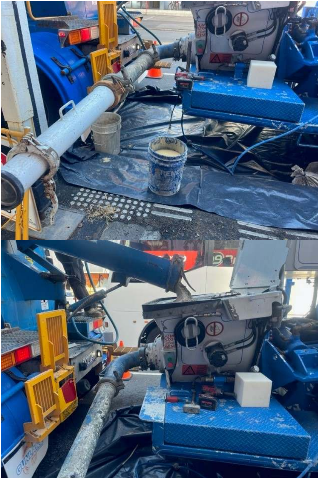
Photos 3 & 4: Concrete pumping was underway with controls in place to reduce the risk of spill release into the street stormwater system.
