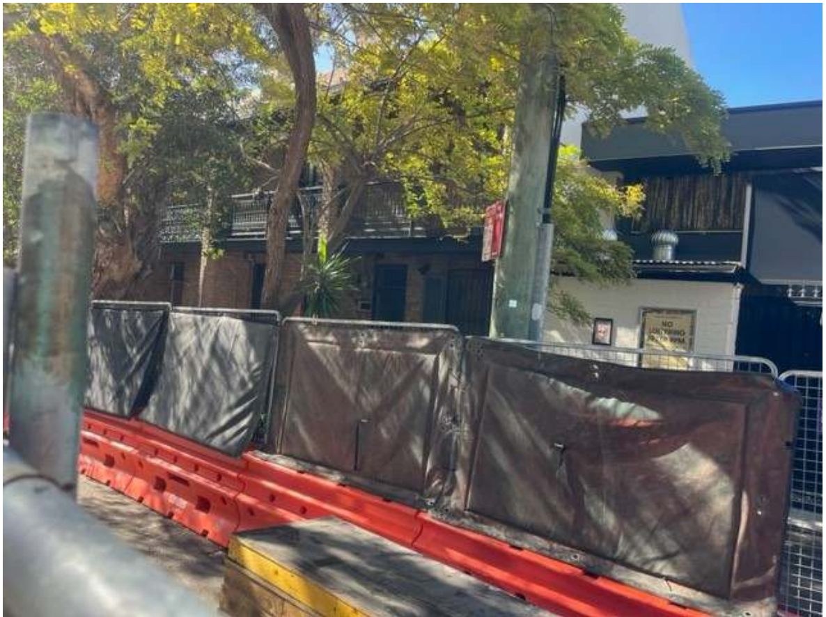
Photo 13: Noise blankets were in place between the work zone and residents on Wellington Street.
