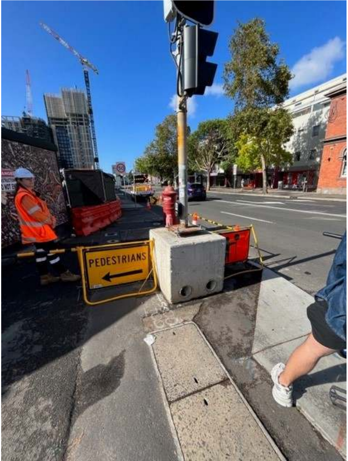
Photo 2: Traffic control and pedestrian diversions in place to allow deliveries in the work zone on Botany Road.
