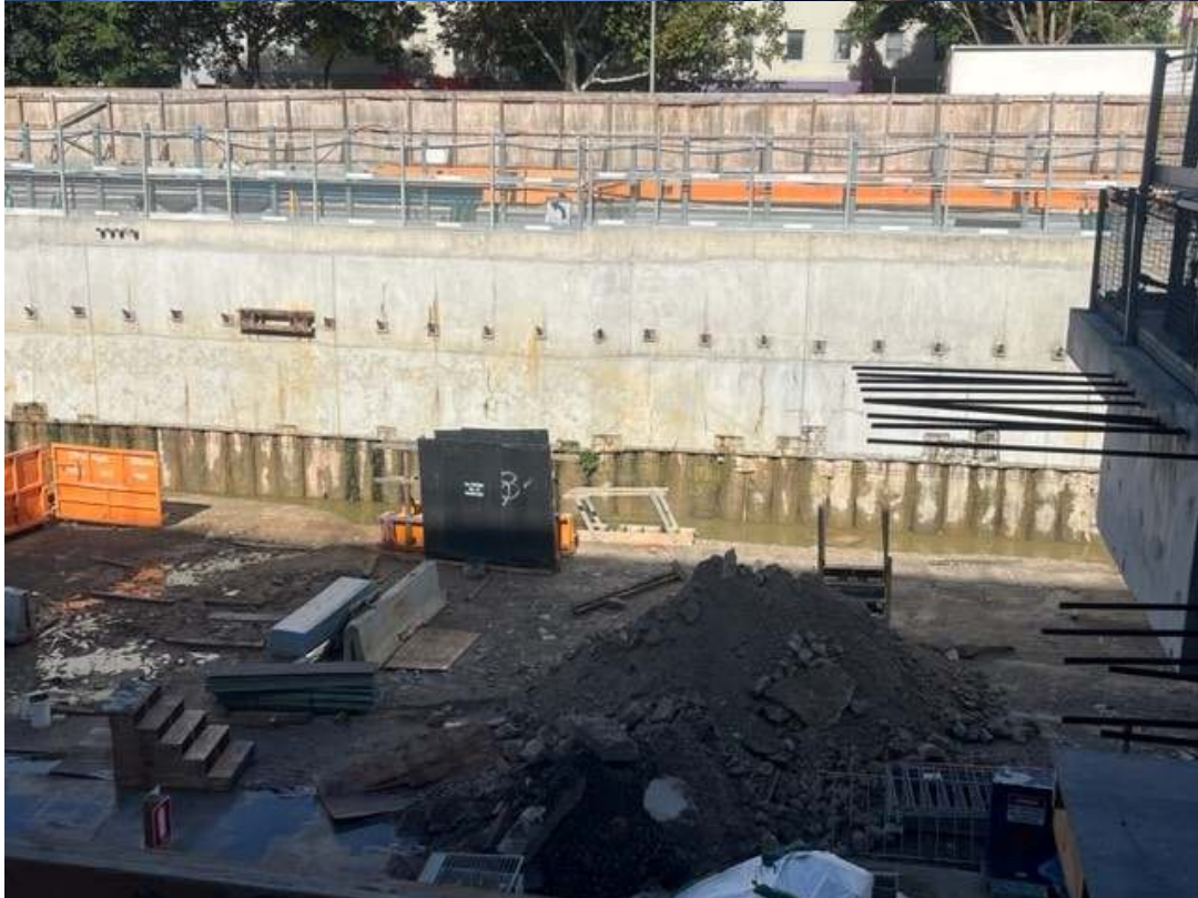
Photos 4 & 5: The last basement slab had been poured and materials were scheduled for removal. Two stockpiles remained.
