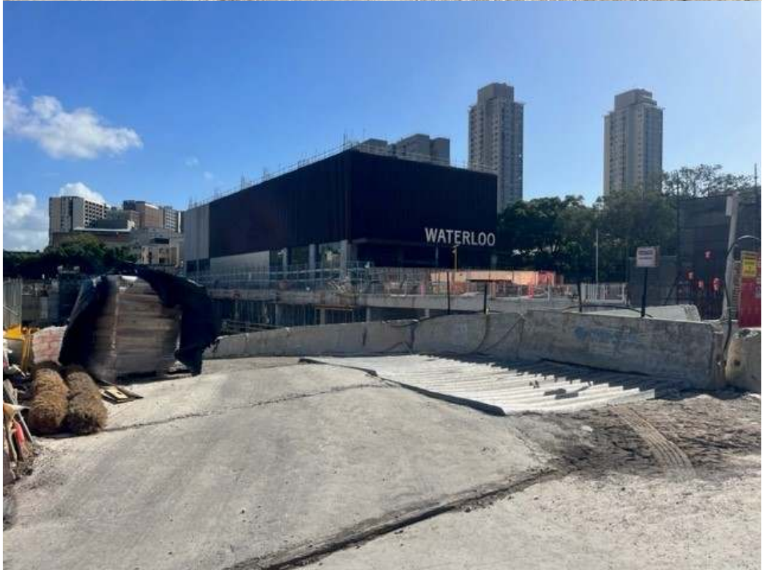
Photos 7 & 8: The rumble grid remained in place for the demobilisation of plant and equipment from the basement. No tracking was observed onto Botany Road.
