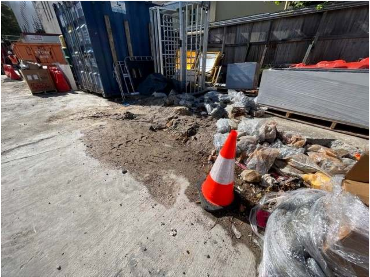
Photo 9: Some excess erodible material and disposal items were observed near the basement access from Botany Road. These items should be removed / cleaned up to reduce potential sediment release from the driveway during wet weather.
