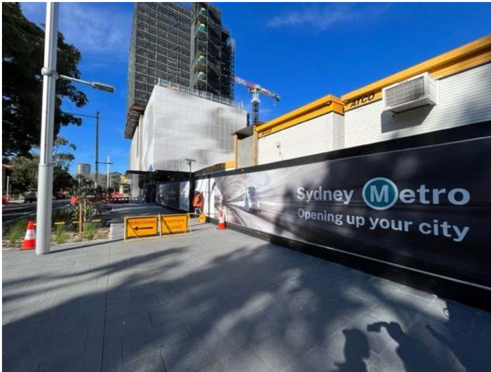
Photo 4: A permit was in place for footpath and kerbside closure to allow for scaffolding removal from Building 4 (Social Housing). The scaffolding would be removed intermittently over 12 days with the footpath reopened as needed in between schedule works. Traffic signage for pedestrian diversion was in place.
