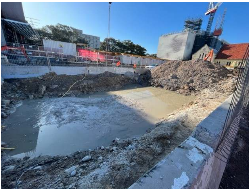
Photo 4: New turkey's nest under construction with accumulated surface water pumped from the old turkey's nest
