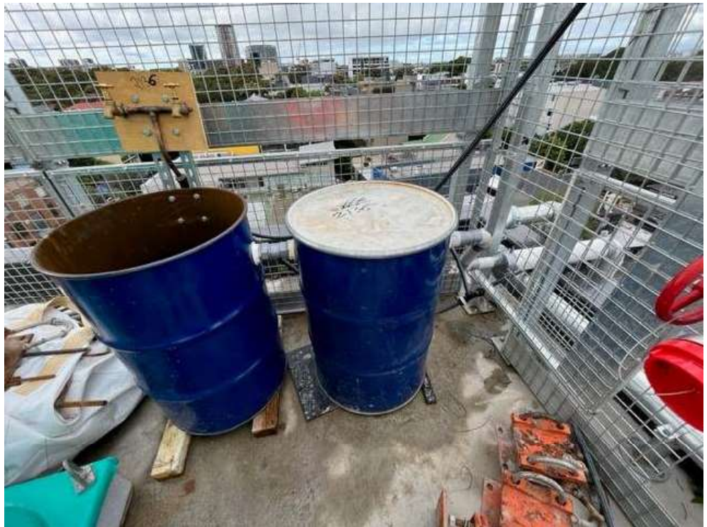
Photo 5: Drums in place for washing concrete hand tools – discharge system to ground floor set up
