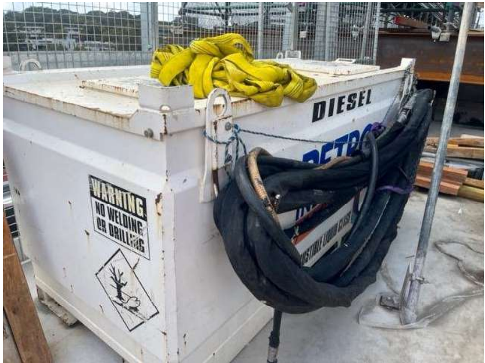
Photo 7: Diesel cell for the crane on the roof of the southern station box
